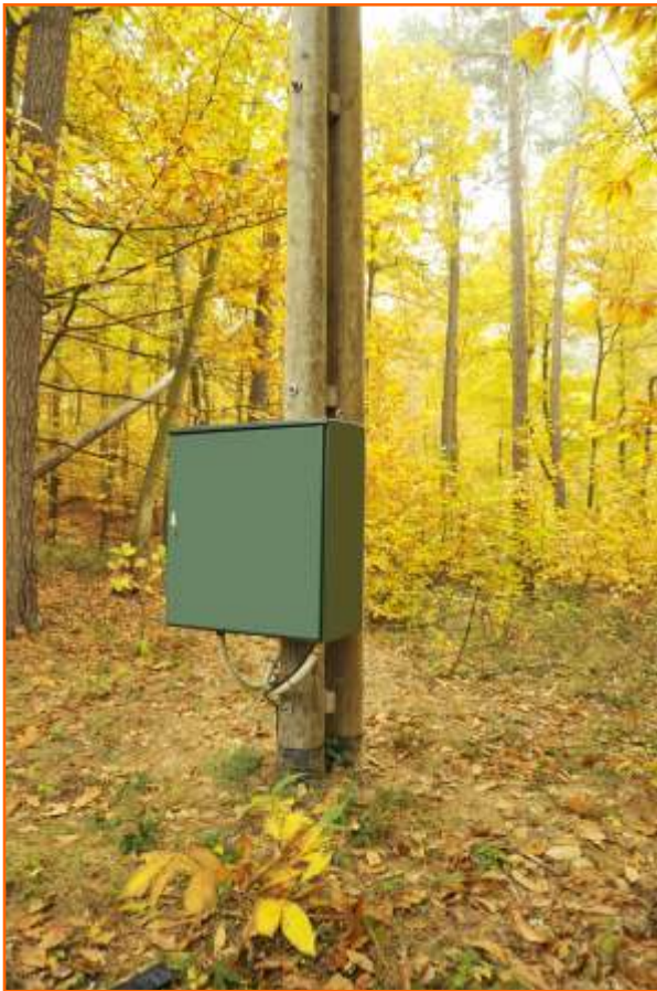
Voltage regulator WA-NRE-M69
