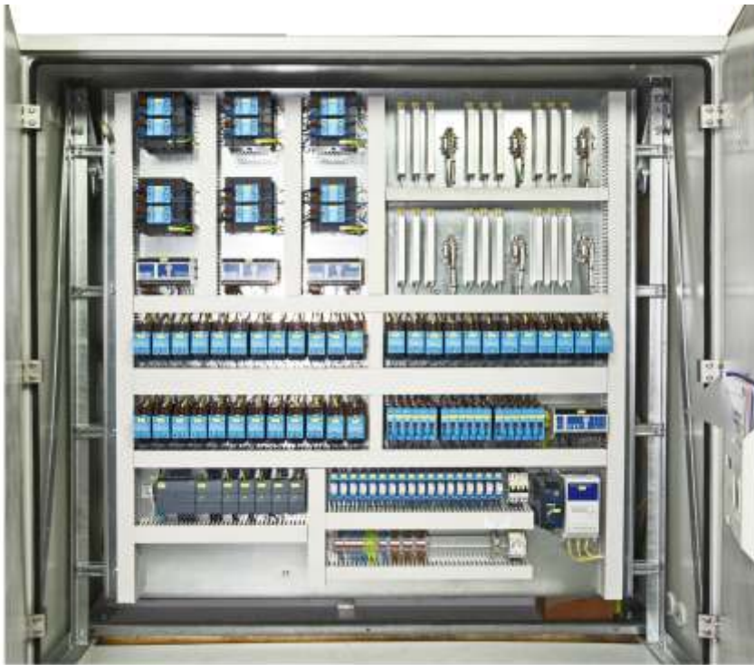
Front and rear view of a 4 door voltage regulator, prepared for installation on a concrete base
